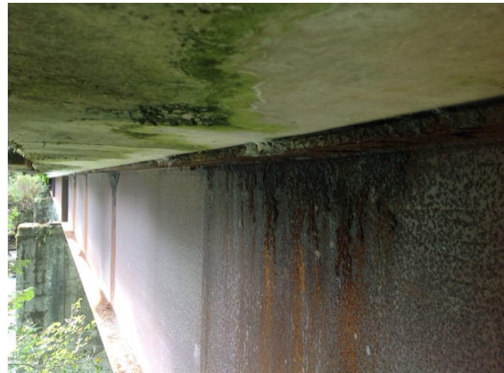
top flange corrosion on left downstream girder
