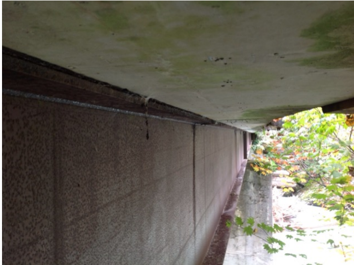
top flange corrosion on left upstream girder - limited to outside of girder
