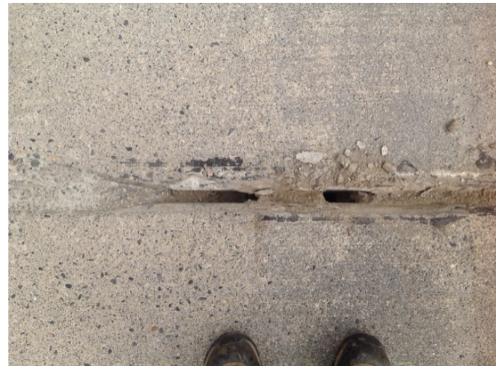
compression seals on both jump spans missing
