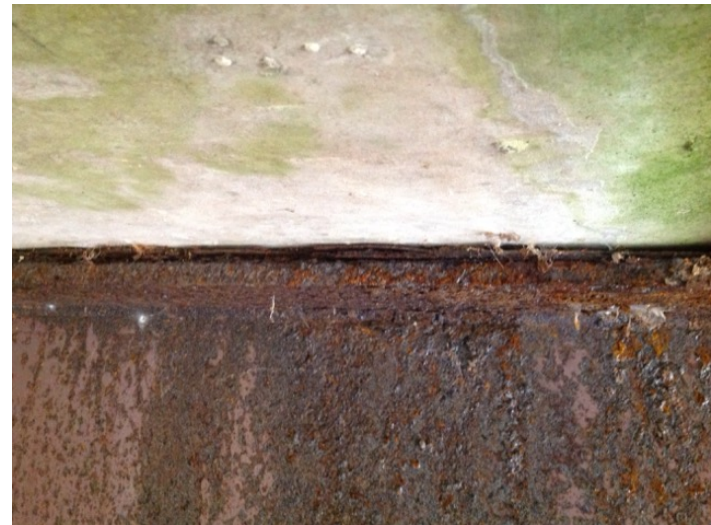
top flange corrosion from poor deck joints
